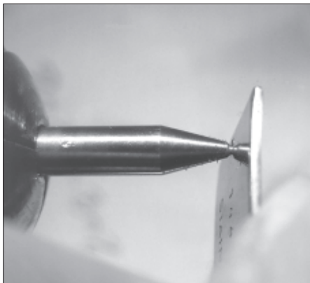
Figure 1. A carbide spade drill was used to drill through the threaded and rusted stud.
